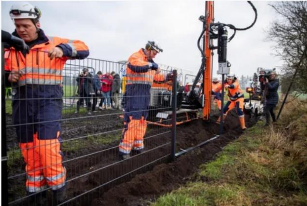
Workers erect a fence along Denmark's border with Germany at Padborg, Denmark, on Monday, Jan. 28, 2019. Denmark has begun erecting a 70-kilometer (43.4-mile) fence along the German border to keep out wild boars in an attempt to prevent the spread of African swine fever, which could jeopardize the country's valuable pork industry. (Photo: Frank Cilius, AP)
